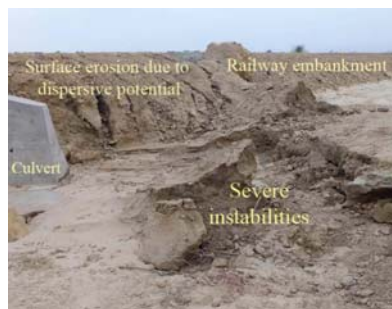
Fig. 2 Severe stability problems occurred at the studied railway embankment after a high rain season during the Spring of 2019
