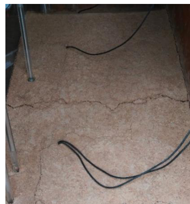
Fig. 17 Main cracks in the middle of the slope
