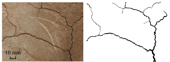
(a) Surface crack image after stabilization (b) Surface crack image after binarization
