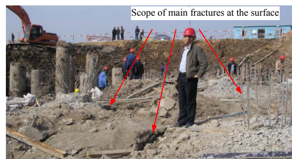
Fig.15 Distribution of surface cracks after excavation of foundation pit
