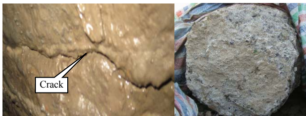
Fig.1 Horizontal crack and section of pile at the crack caused by excavation
