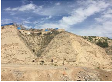
Fig.24 A section of Shigou unstable slope
