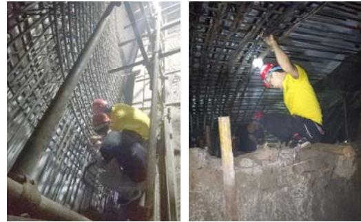
(b) Construction drawing of optical fiber layout in secondary lining Fig.12 Optical fiber layout position and construction drawing in second lining
