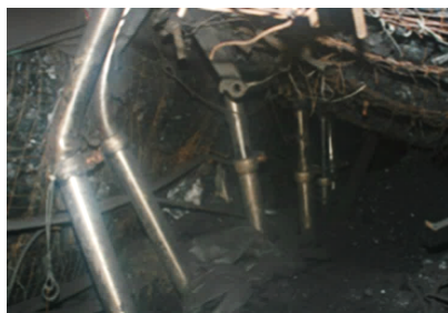
Fig. 5 Scene of roadway support failure impacted by the roof
